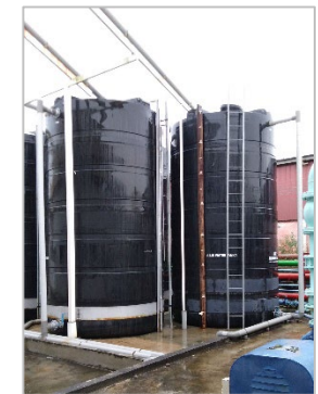
SMM's rainwater tanks
