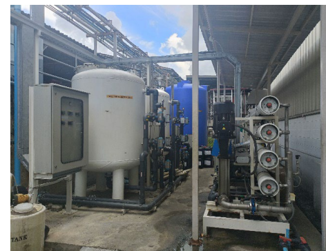
SATL's water recycling equipment
